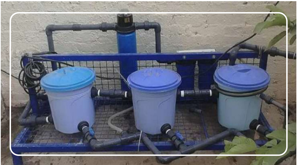
Cairo University owns a pilot wastewater treatment plant for the safe disposal of wastewater
